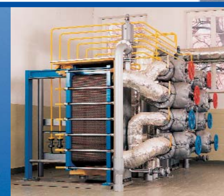
District heating system
